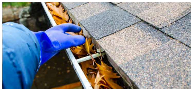
Figure 10: Example of debris accumulation in gutter
