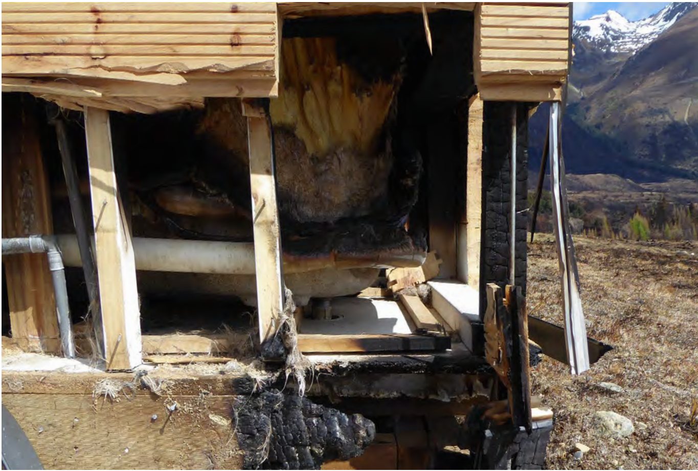
Figure 12: Example of how vulnerable timber cladding is to ember attack, radiant heat or direct flame. Fire has broken through and set bathroom inside alight. Ōhau 2021 (Fire 3088958)
